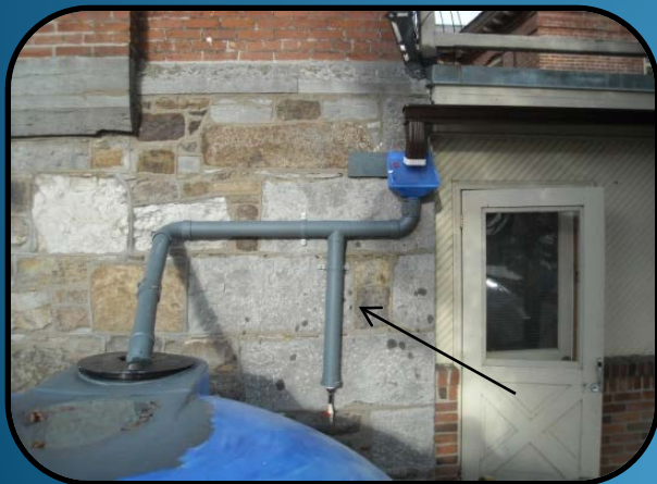
First flush contaminant catchment
