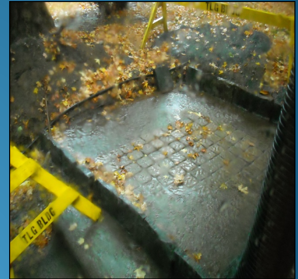
Rain water accumulates on new cistern containment pad
