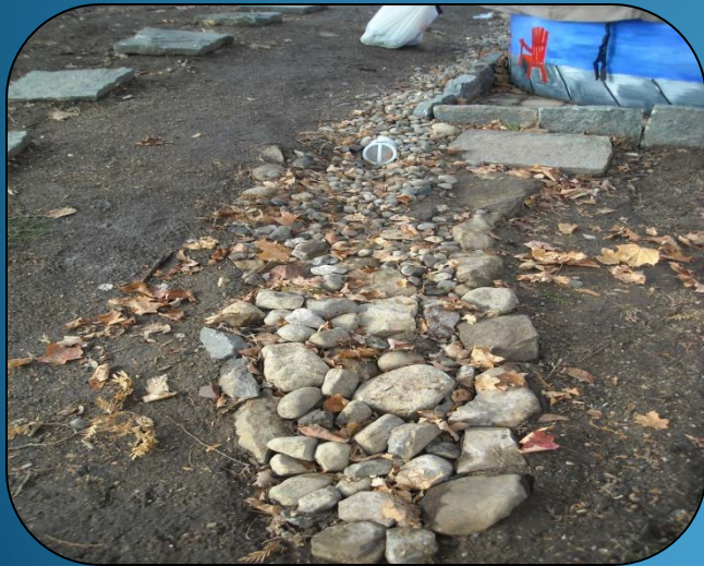
Overflow discharge and rock-lined absorption
